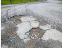
Potholes on asphalt road 20171023.j... commons.wikimedia.org
